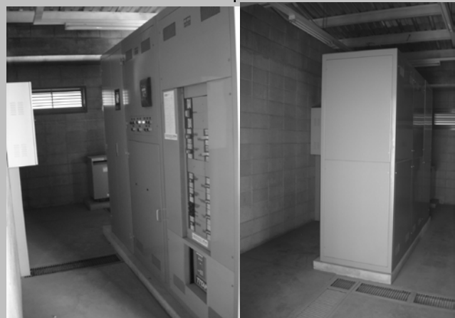
Sala Tablero Principal
