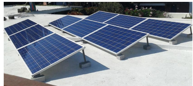
Figura 8.5: Panel fotovoltaico, ALTERNATIVE, Solar Energy 2014.
