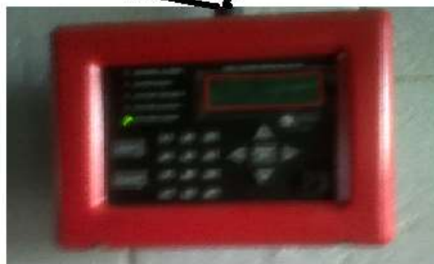
Panel de control
