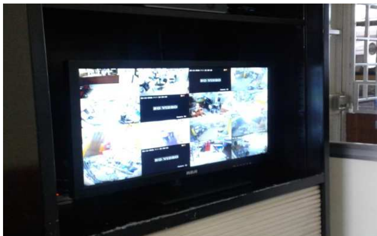
Panel de control principal
