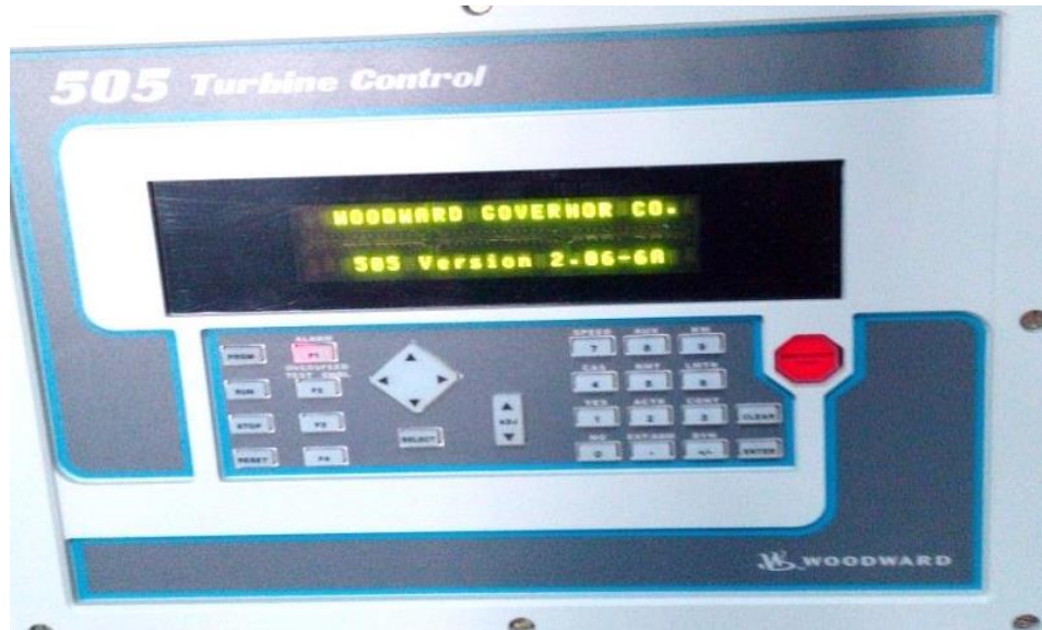
Figura 35. Tablero de control Woodward 505
