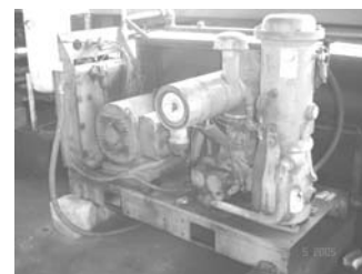
No. 3 Compresor Quincy
