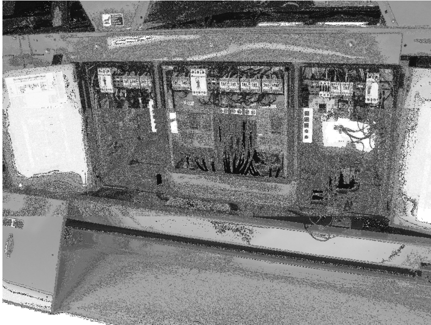
Figura 42. Panel de control, chiller 30XA200
