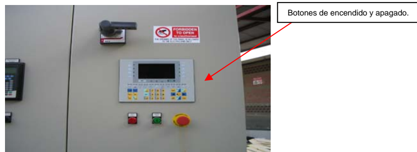
Figura 8. Panel de control
