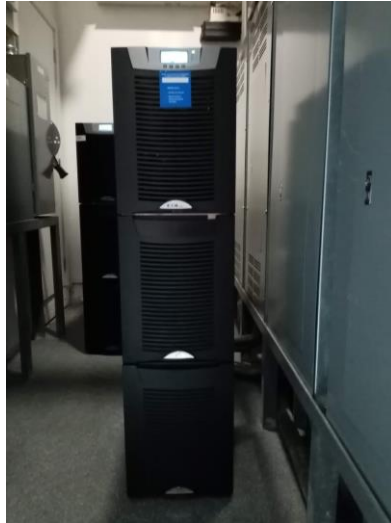
Figura 9. UPS ( Uninterruptible Power Supply )
