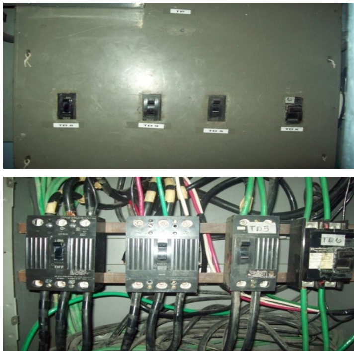
Figura 15. Tablero Principal (TP)
