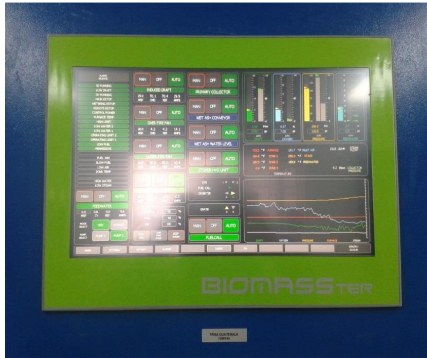
Figura 23. Panel de control Biomaster
