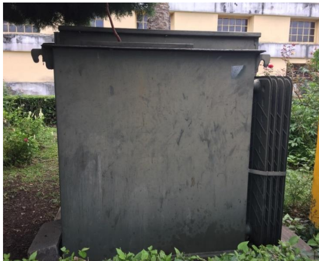
Figura 4. Transformador Pad Mounted
