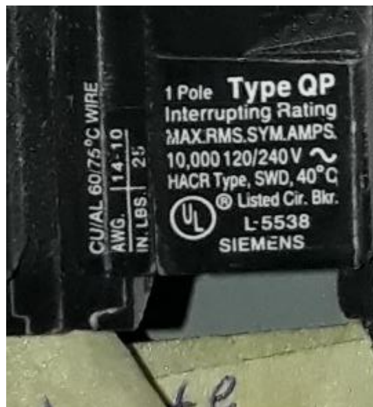
Figura 44. Breaker principal MUNAE
