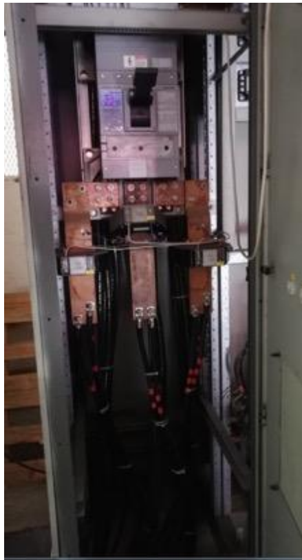
Figura 55. Interruptor principal, celda 1
