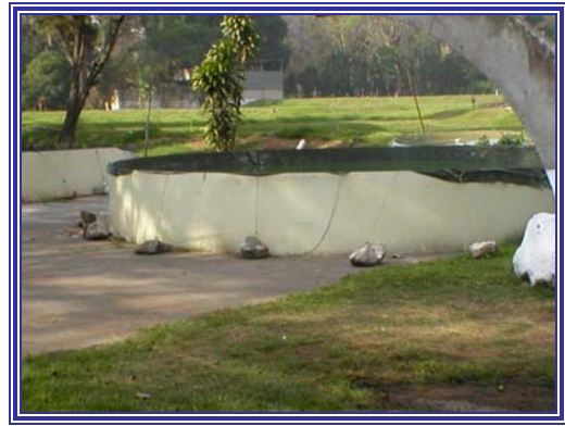
Figura No. 5 Tanques circulares
