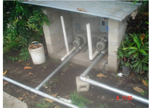
Figura No. 63 Blowers
